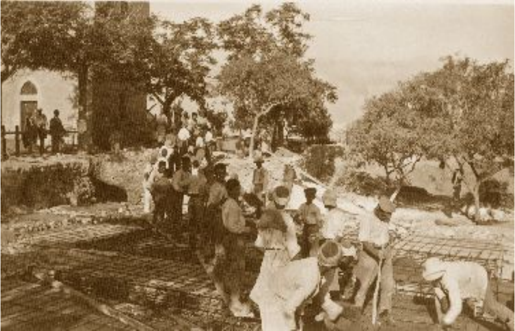
Spring 1928: young people help in the casting of the slab above the crypt.
