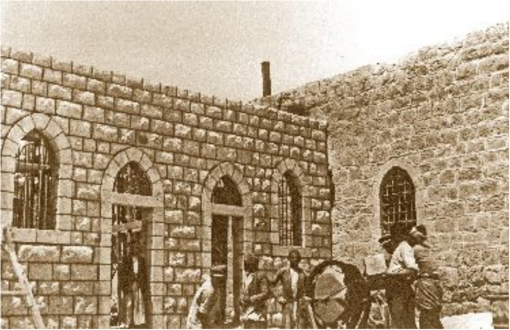
Bro. Srugi, covered by the man mixing cement, closely follows building works.
